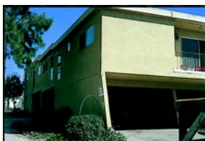
Ground story near-collapse of an apartment building in the 1971 San Fernando Earthquake. The structural problem is the same as surfaced in the 1994 Northridge Earthquake: Inadequate ground story earthquake resistance on the side where the parking stalls are located.
