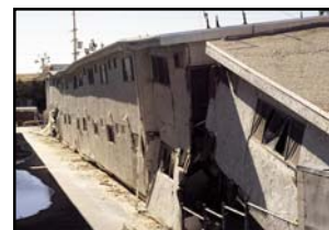
Ground story collapse, 3-story apartment building, 1994 Northridge Earthquake
