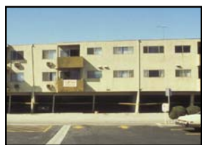
This view of an apartment building that leaned over but did not quite collapse in the 1994 Northridge Earthquake illustrates the excessive sidesway at the ground story parking area, which in combination with the large weight from stories above, can cause the ground story to collapse.
